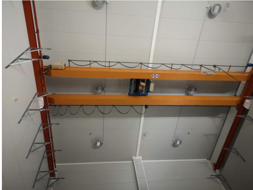
Figure 10: the BIH overhead crane (3.2T maximum load capacity)
